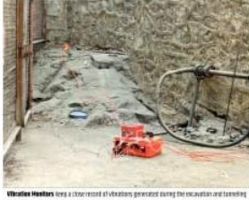
Vibration Meters keep a check on vibrations generated during the excavation and tunneling.
