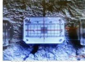
Crack Monitoring Meters are installed across a pre-existing crack to measure if any expansion takes place in the crack.
